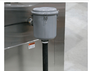
External filter protects vacuum and room from dust.
